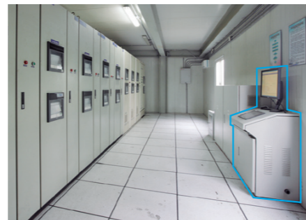
Fig.2: Considerably-miniaturized process management system for a forging furnace. The equipment on the left in the picture is the existing system with pen recorders. The terminal of the new control system using CC-Link IE is on the right in this picture.
